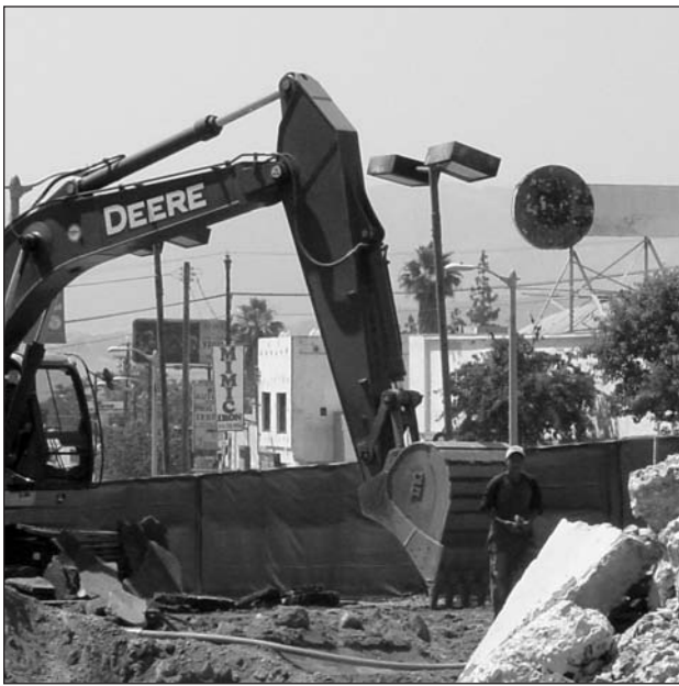
Asphalt being removed in preparation for new center with restaurants and retail shops on old Ford property at the corner of Foothill Blvd. and Commerce Ave. in Sunland-Tujunga.
